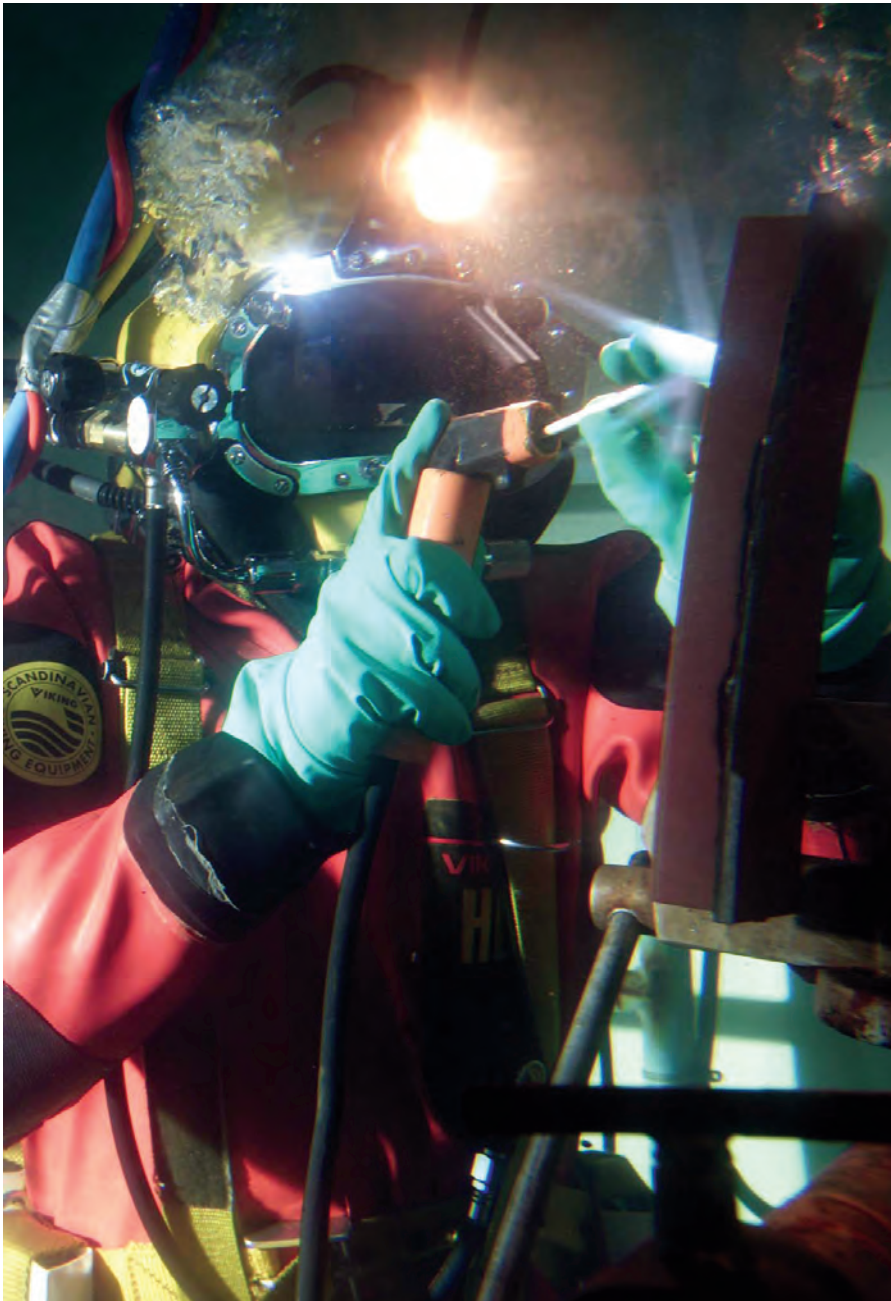
Fig. 1 — Welding for qualification test in tank with full diving gear. (Courtesy of the Royal Dutch Navy — Diving Group.)
